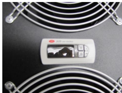
User set point control, display for Rack Face Temperature
